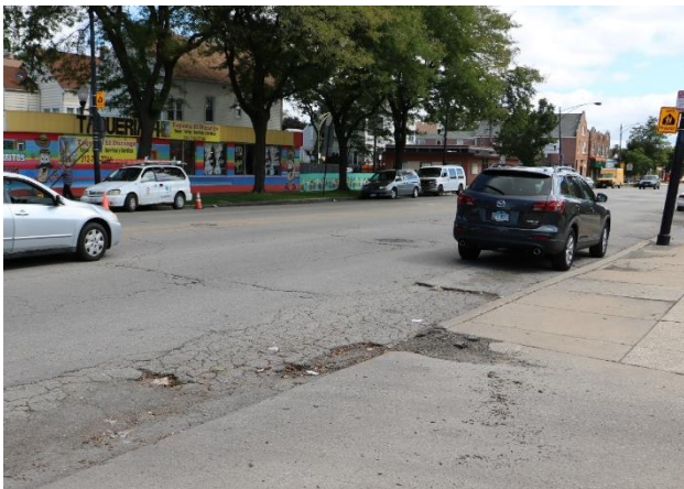
Deteriorated pavement and sidewalk along Fullerton Avenue
