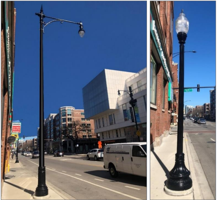
New decorative street lights
